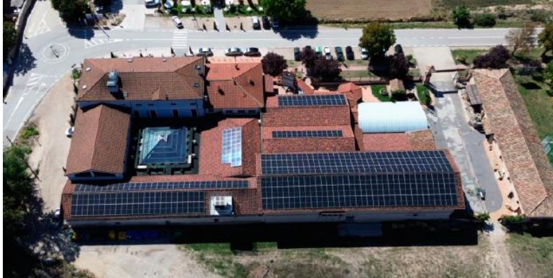
Bodegas Lagar de Isilla. 192 KWp photovoltaic self-consumption plant in Castilla y León.
