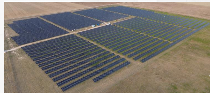
Villanubla Solar Plant 10.39 MW photovoltaic plant Castilla y León, Valladolid
