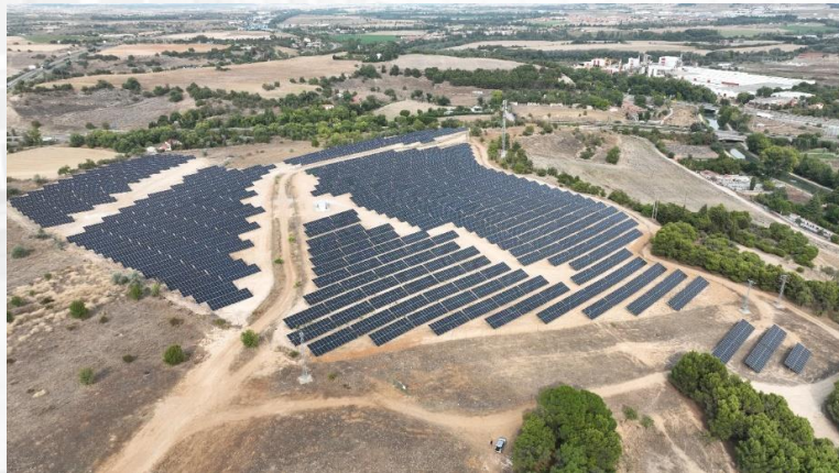
Industrial self-consumption PV installation on the ground. Lingotes Espaciales SA. Capacity of 5.9 MW. Finished in July 2024. Castilla y León.
