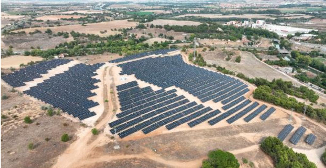
Ground-mounted photovoltaic installation for industrial self-consumption for Lingotes Espaciales SA. Power of 5.9 MW in Castilla y León.
